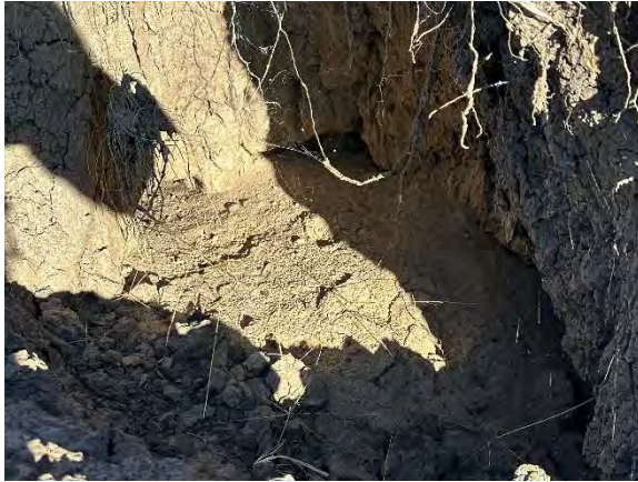
Figure 3-2 Hollow in erosion bank
