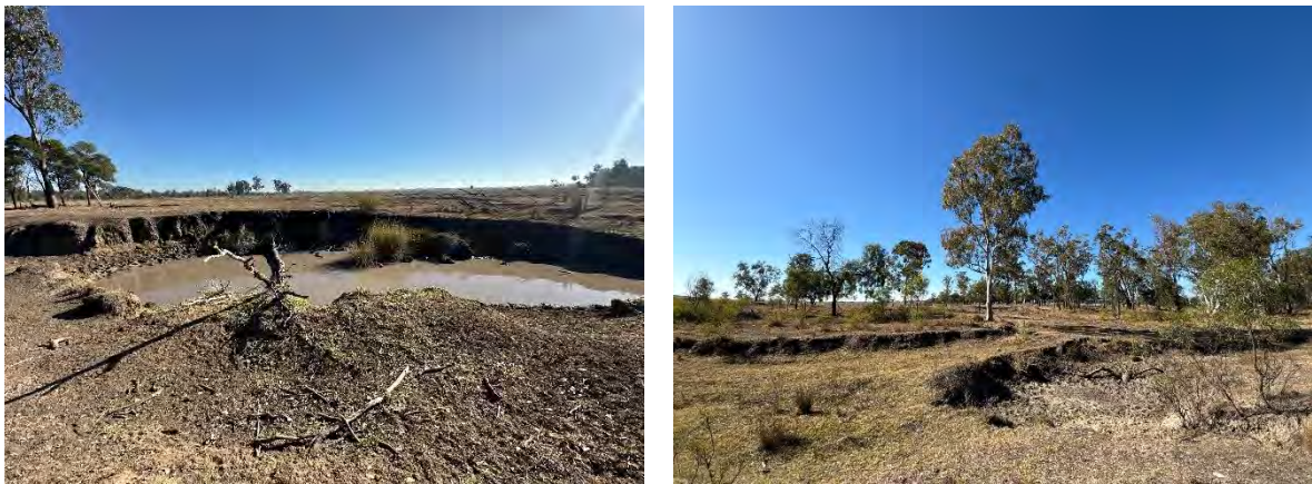
Figure 3-5 Examples of erosion on creek bank
