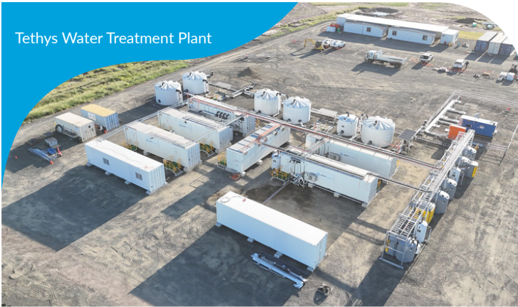
Brine storage at Tethys plant
